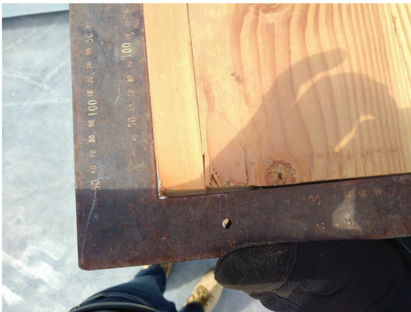
Slight compression deformation at the rocking wall corner
